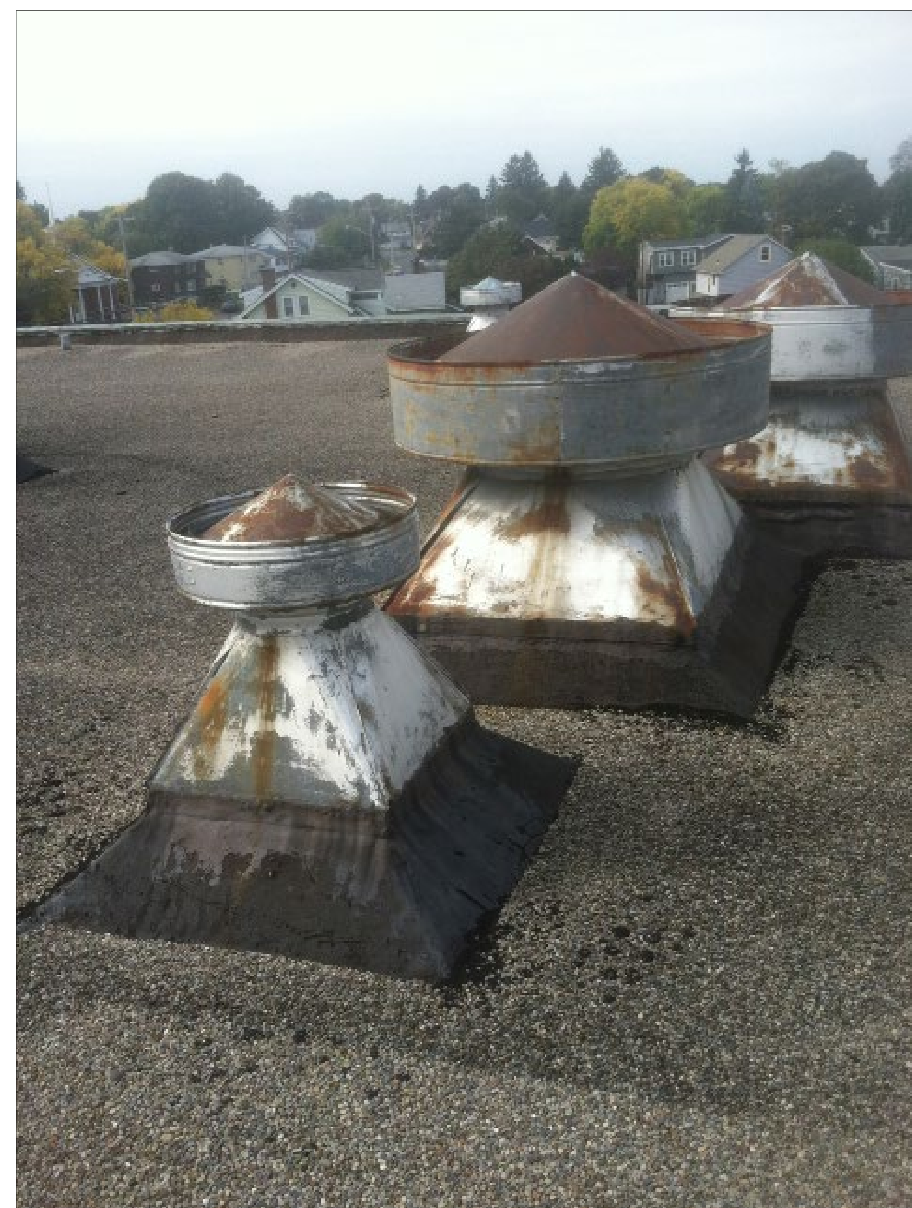
ROOF TOP VENTILATORS
