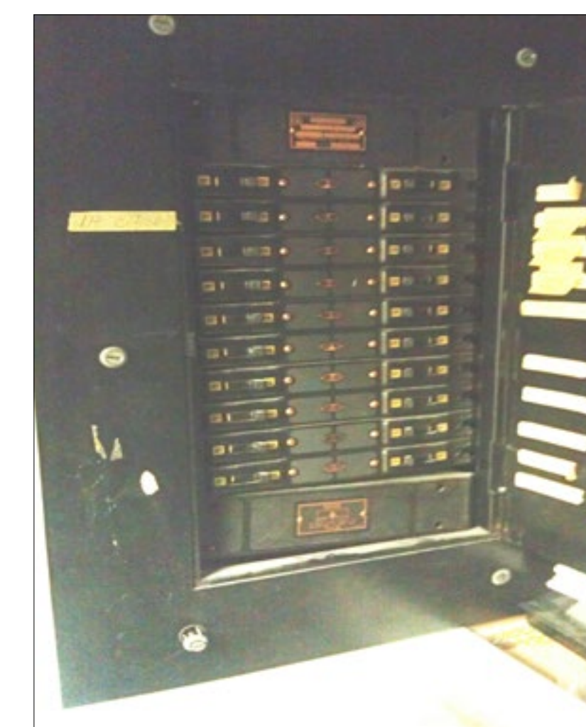
OLD ELECTRIC PANEL
