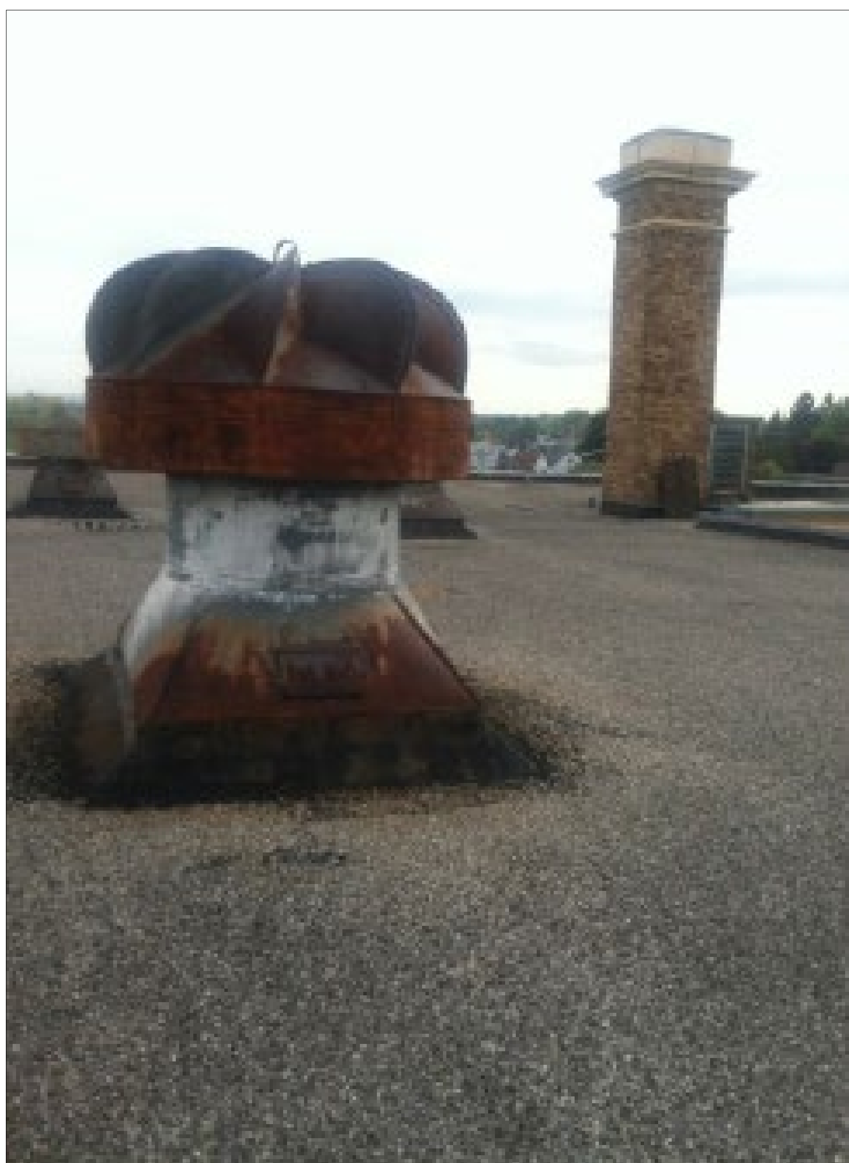
ROOF TOP VENTILATORS
